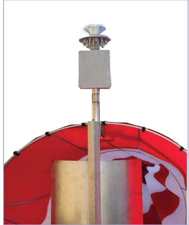
LED Obstruction Light Fitted above sock
